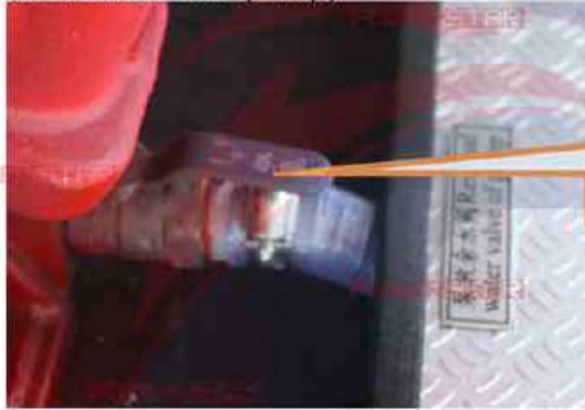
Residual Water Valve of Pump
